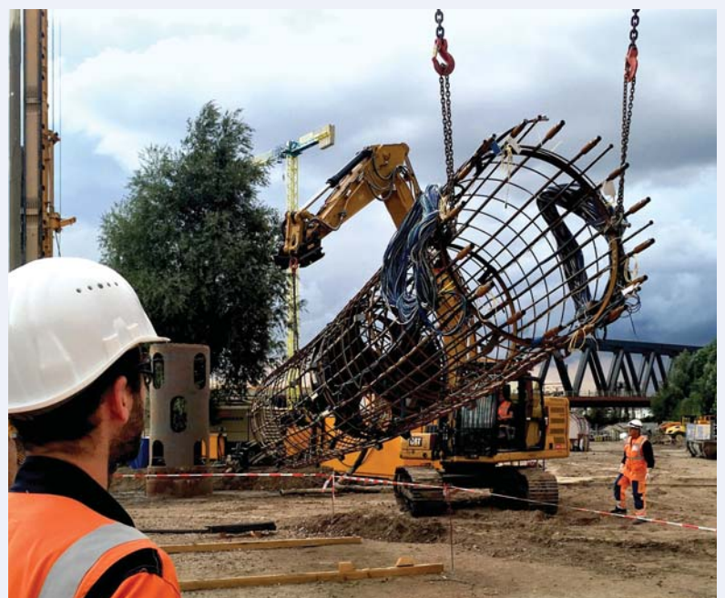
Photo 2 – Photo 2: BAUER Spezialtiefbau GmbH verified the foundation design for a more cost-efficient and less time-consuming solution.
