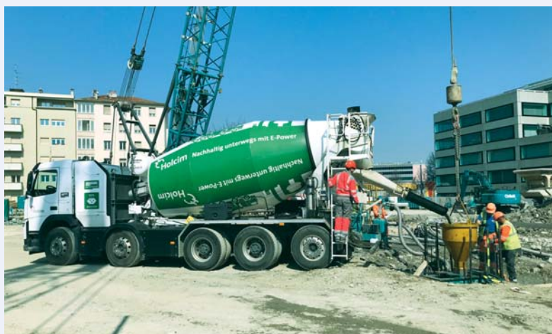
Photo 1 – Construction work in Geneva; the carbon footprint on the project was reduced by one third (420 tonnes) using, among other things, electric concrete trucks.
