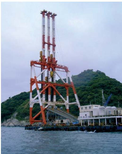
Soil improvement with SCP process at the western end of the tunnel.
