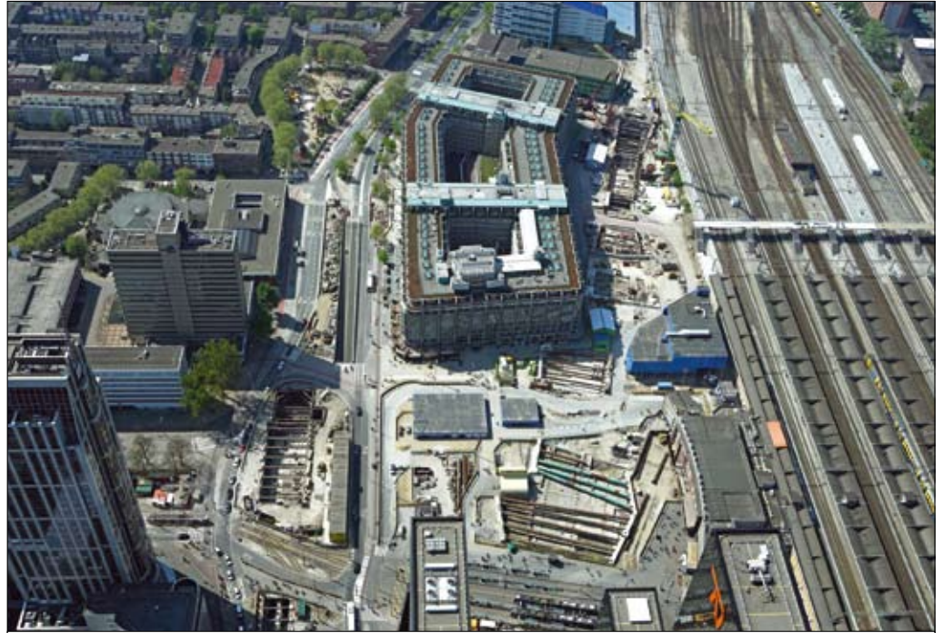
↑ Figure 4 Work in progress. Left: the building pit for the new Weenatunnel. Right in front: the building pit for the underground metro station CS. Right at the back: the building pit for RandstadRail, including the end shaft (photo Aeroview)
