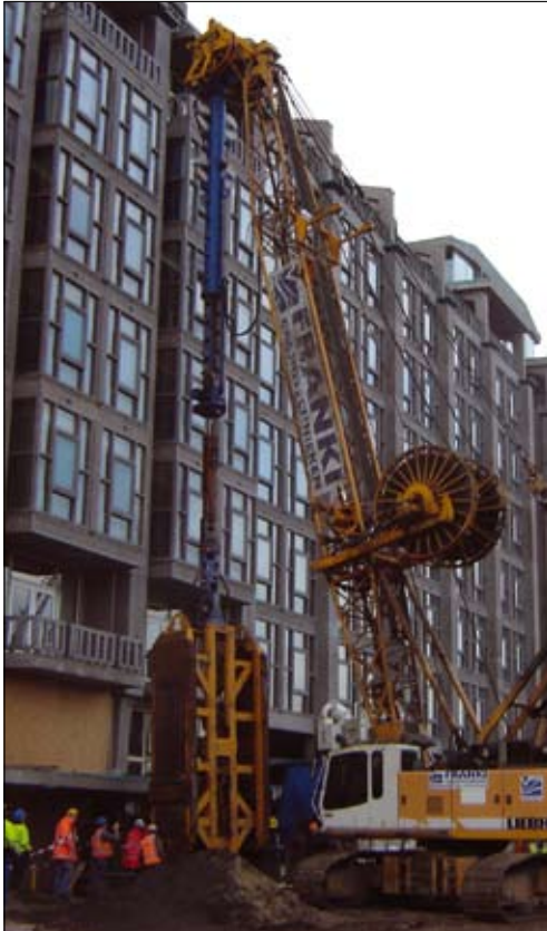
↑ Figure 5 The installation of diaphragm walls next to the Groothandelsgebouw (photo Aeroview)
